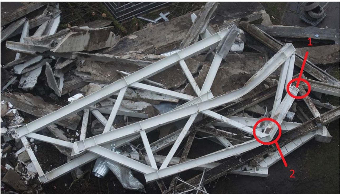
Figure 6. Tension connection ( 1 ) has failed from bolts just as theory would predict. Connection ( 2 ) has failed during the collapse, since this diagonal is in compression and does not fail or fracture in normal compression loading conditions. Only tension bars and connections rupture.
