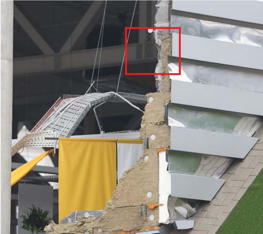
Figure 1. Truss bottom chord is connected with end plates and bolts which are in between steel beam flanges. The quantity and sizes of bolts are not sufficient for massive steel beam section. Bolts should also be placed outside of flanges (see figure 5 for example)
